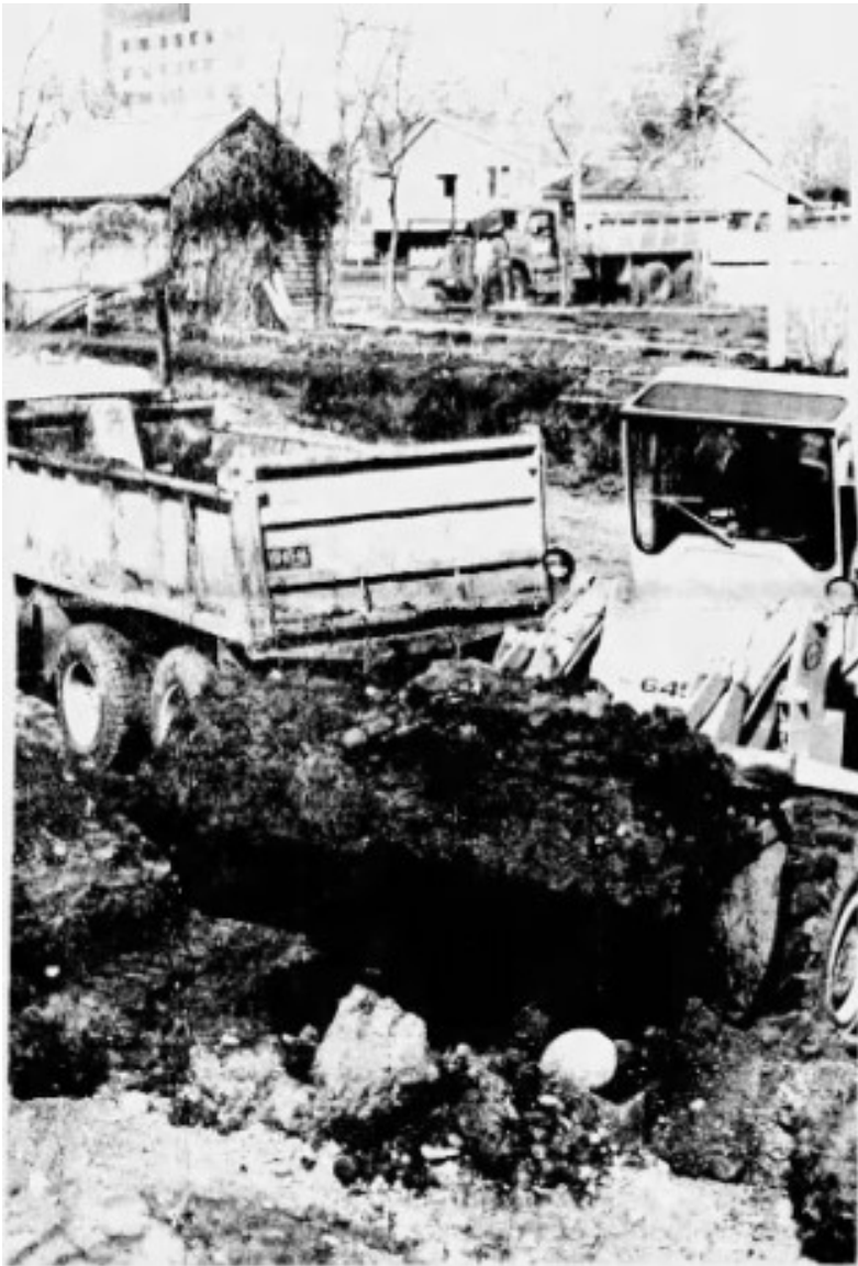
A front-end loader takes another bite as it digs out the basement for Grande Prairie's new movie theatre and billiard hall.
